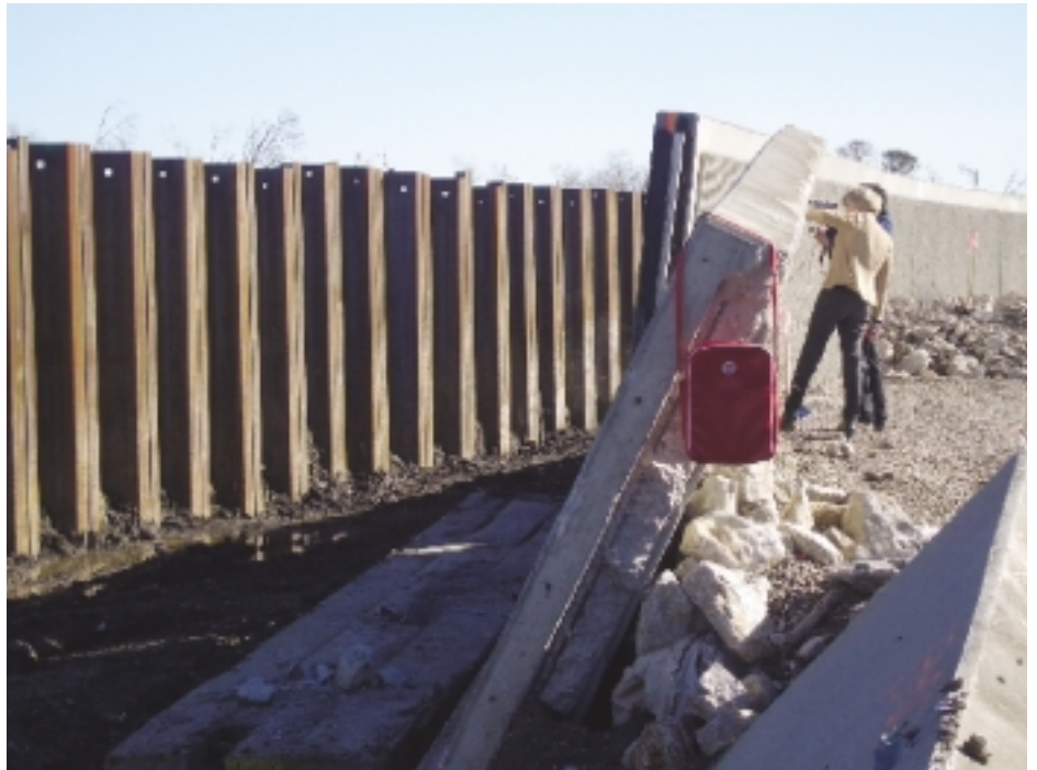
The London Avenue Canal breach
